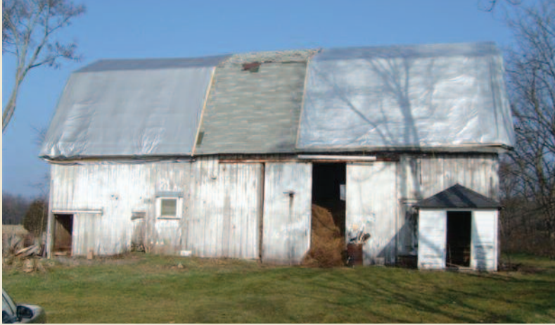
Jones tarped holes in the roof to allow the barn to dry inside while hay and clutter were cleaned out in preparation for dismantling and moving.
