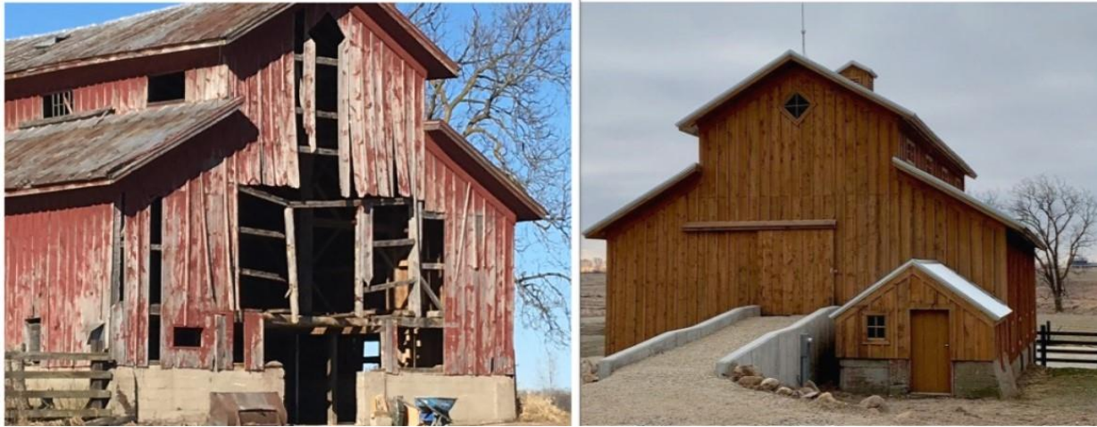
Prairie Bells Barn, a new event venue northeast of Grand Rapids, before and after renovation.
